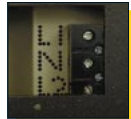
One electrical hook-up
